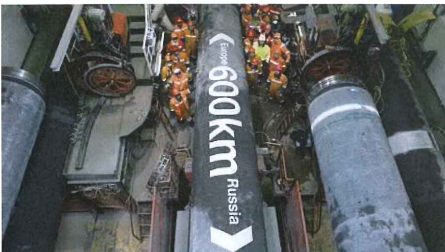
Nord Stream 2 would largely run along the same 1,224 km route as the existing Nord Stream. (Nord Stream)
